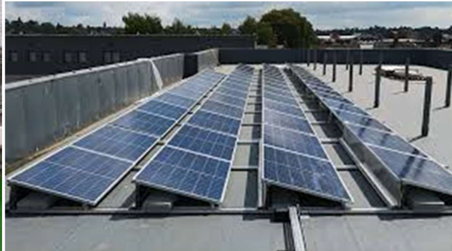
Photovoltaic Panels on the roof of City Hall
